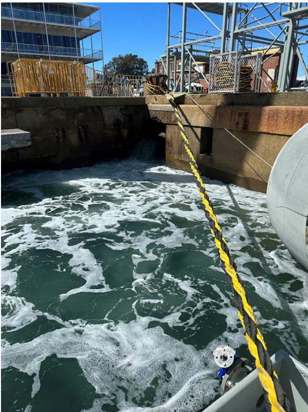
Outflow from the CCD pumps (Photo courtesy Sean Langman)
