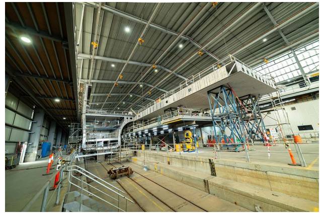
A stern view of Incat Hull 096 under construction (Photo courtesy Incat Tasmania)
