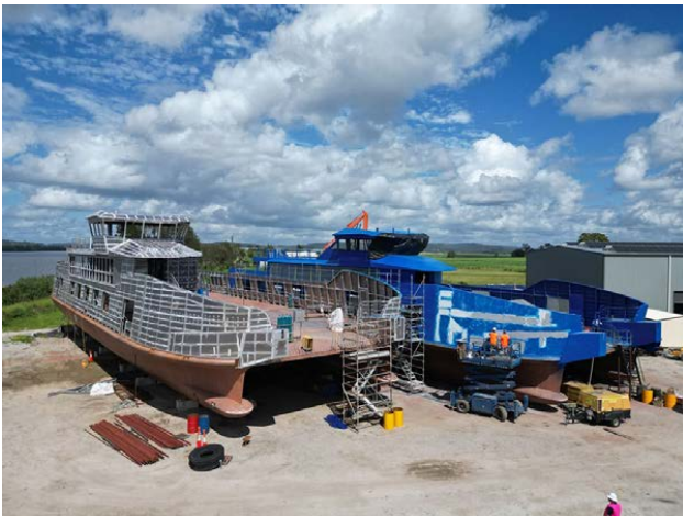
Mirrabooka and Yarabinjara under construction at Polaris Marine Dockyards, Harwood (Photo courtesy Chris Briggs)
